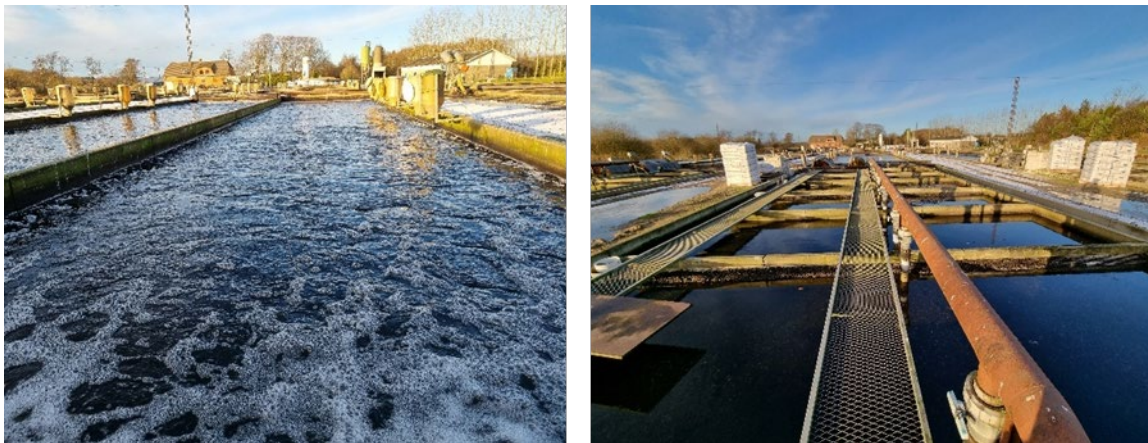
Figure 4-7. Pictures of Nr. Vium Dambrug, with a fish section on the first picture and the fixed bed biofilter section on the second
