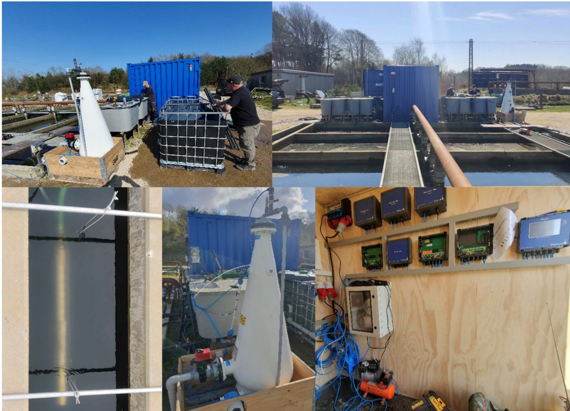
Figure 5-4. Ozonation set-up on a model 3 pond farm. The container, the tanks, the biofilters, feeding pump, the Gaia ozone generator, and the OxyGuard Pacific control systems that were used in the experimental trial can be seen.
